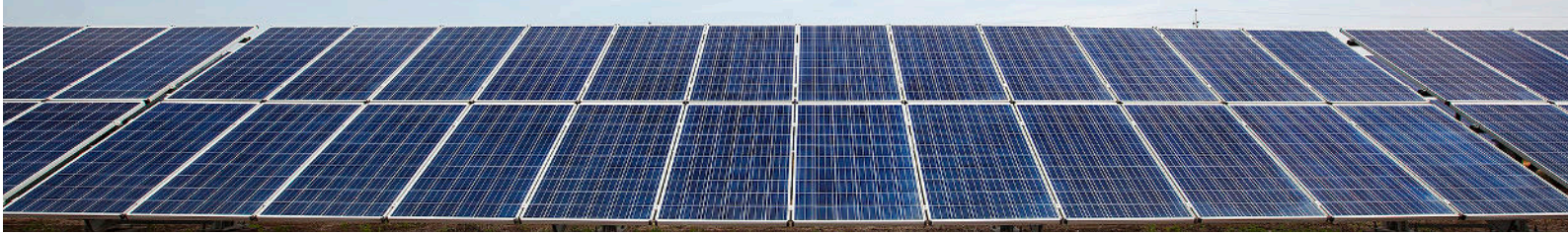
100 MW Solar Park, Zaheerabad, Telangana
